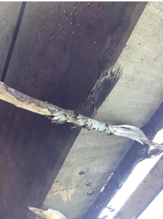
Minor chip upstream girder
